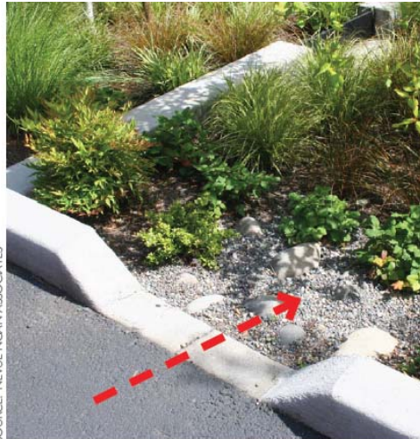
Figure 5-2: This standard curb cut at parking lot rain garden has 45 degree chamfered sides.
