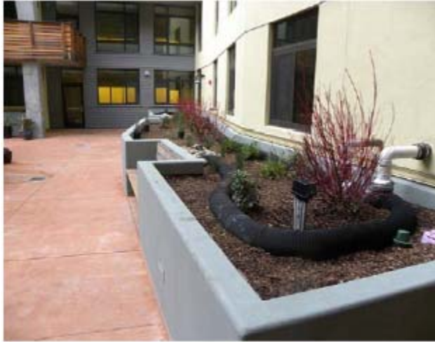
Figure 6-12: Half-buried, perforated flexible pipe serves as a flow spreader to distribute stormwater evenly throughout a long flow-through planter in Emeryville (Source: GreenGrid/Weston Solutions).
