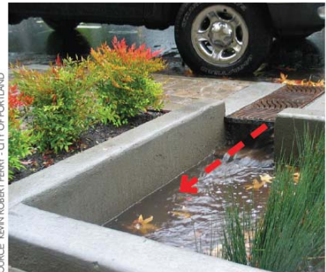
Figure 5-11: A grated curb cut allows stormwater to pass under a pedestrian walkway to the stormwater facility.
