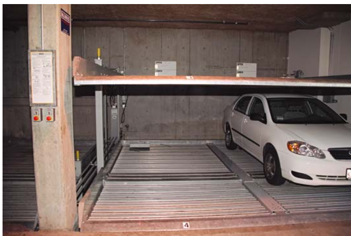
Figure 4-7: Parking Lifts in Parking Garage, Berkeley
