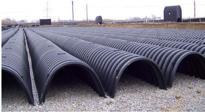
Figure 6-21: Photo of subsurface retention/infiltration system installation under a parking lot. Source: Contech.
