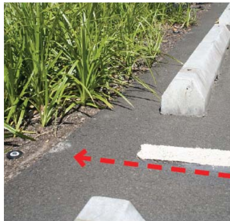
Figure 5-8: Stormwater runoff enters the stormwater facility through the 3-foot space between these wheelstops. The design could be improved by providing more of a drop in grade between the asphalt and landscape area.
