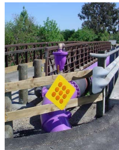
North Bayshore is served by a recycled water system.
