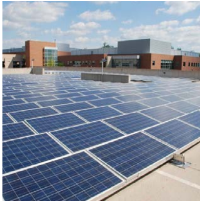
Rooftop solar panels in North Bayshore.
