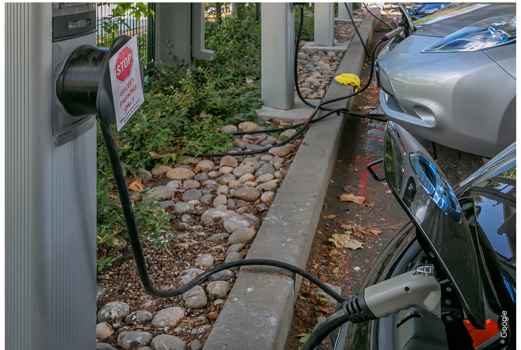
Figure 5.6.1. ELECTRIC VEHICLE CHARGING STATIONS
