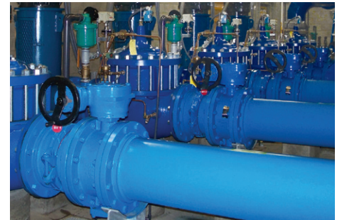
Graham Reservoir Pump Station
