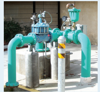
City groundwater supply well
